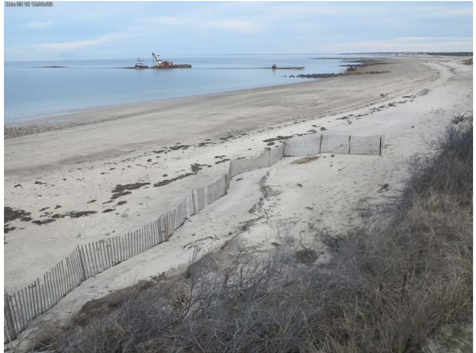
A view from the beach cam on Christmas Day 2015 shows tugs and barges working to install the sand delivery pipe.
