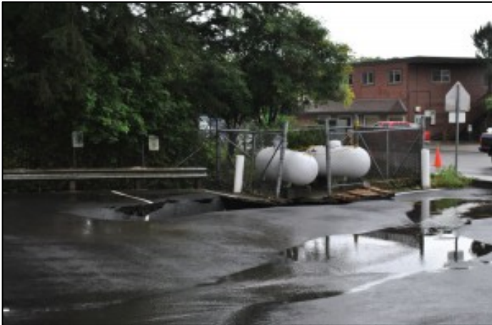
Photo 1- A sinkhole had opened up beneath a pair of propane tanks on Halibut Point Road. (Rebecca LaGuire, KCAW)
